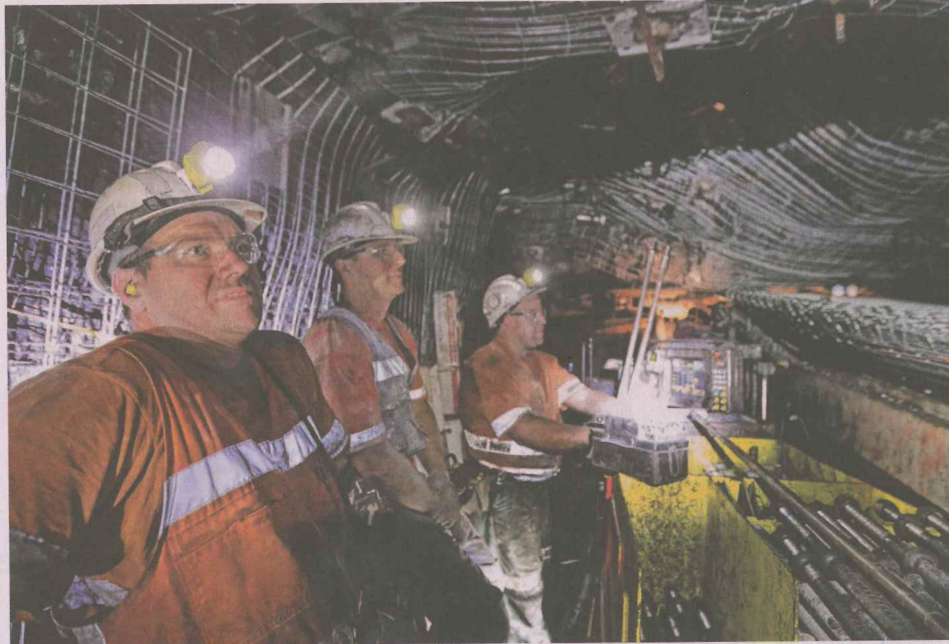
Workers bore into the coal seam to create an access tunnel for the longwall miner at BHP's Broadmeadow underground mine
